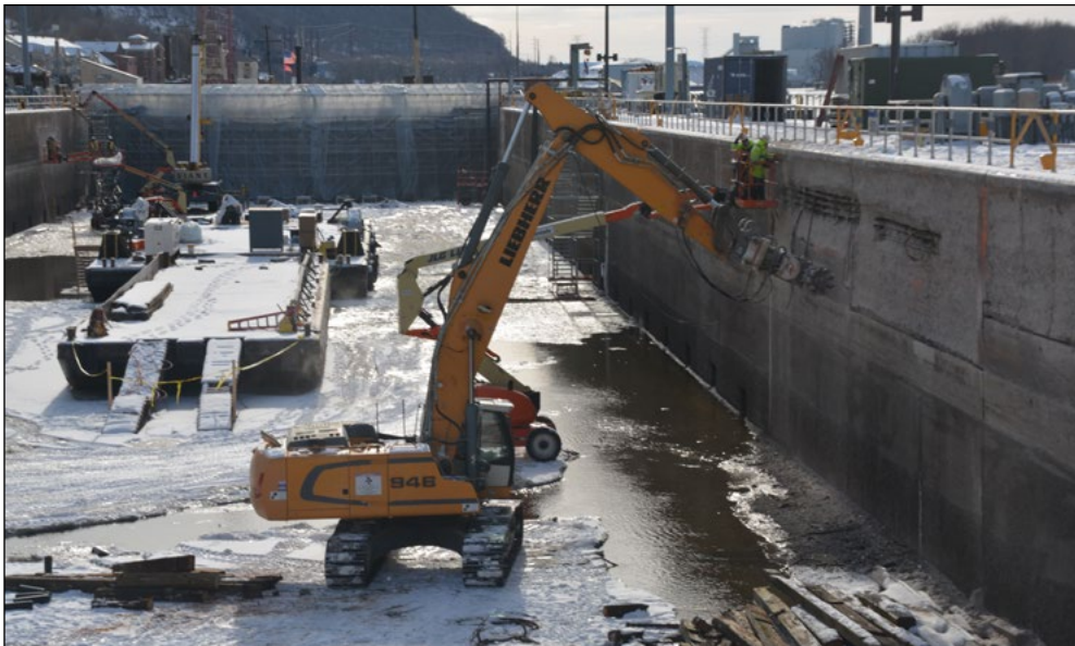
The lock chamber at Lock and Dam 4, near Alma, Wisconsin, is dewatered to perform maintenance and repairs. USACE photo by Melanie Peterson
