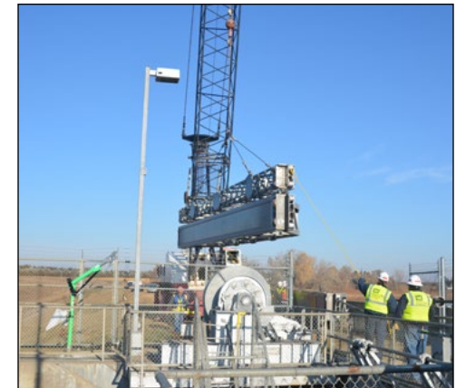
Steel bulkheads are lowered into the water to shut off the spillway so engineers can open and close the dam gates, Nov. 5. Photo by Elizabeth Stoeckmann
