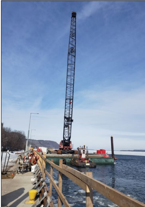
The contractor works to complete tow rail repairs at Lock and Dam 5 near Minnesota City, Minnesota, Feb. 26. USACE photo by Melanie Peterson
