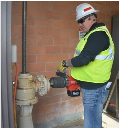
John Fromuth, Orwell Dam site maintenance lead, uses a specialized tool to open and close the dam's lock chamber located, Nov. 5. USACE photo by Elizabeth Stoeckmann
